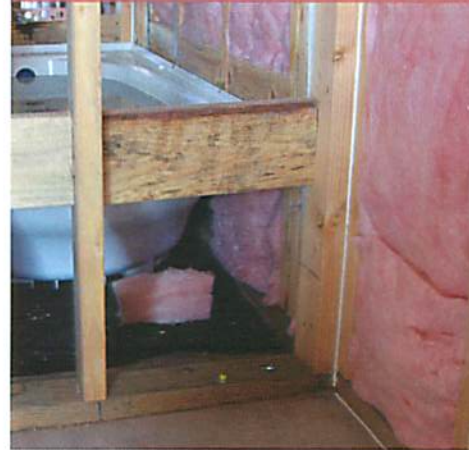
✗ NO RIGID AIR BARRIER
