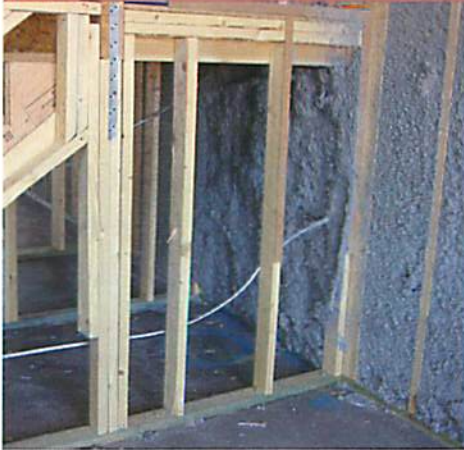
✗ NO RIGID AIR BARRIER
